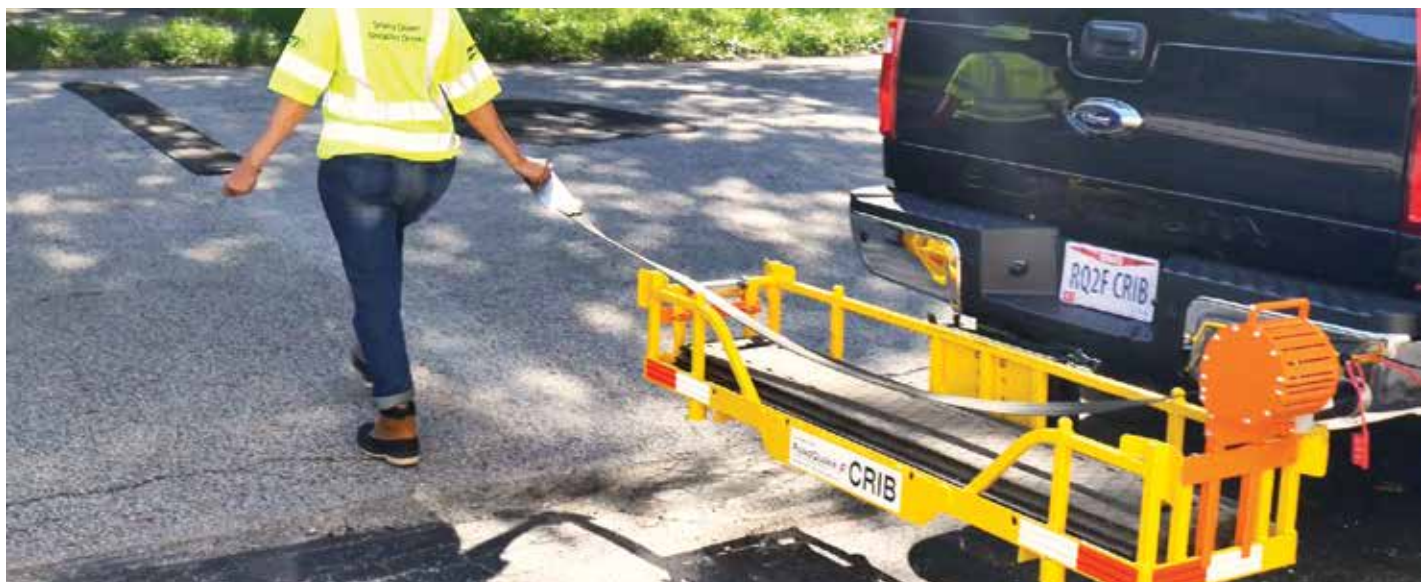
3. Always use caution when working in and around live traffic. Pull Retrieval hook out to the rumble strip array.
